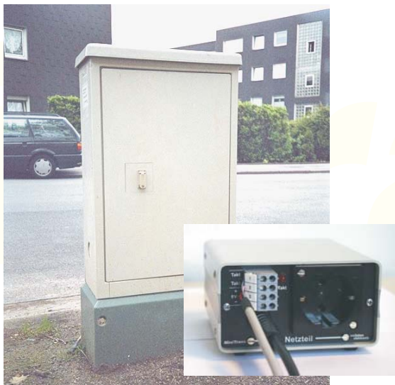
Remote controlled switching of rectifier system with mains power supply unit
